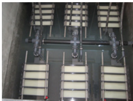
One of two tanks retrofit with Micron Nadir MBR Bio-Cel membranes
